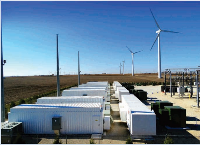
20 MW energy storage solution with NextEra in Illinois, USA
